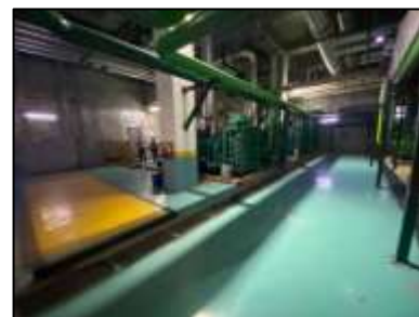
View of DG Room
