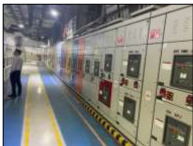
View of LT Panel Room
