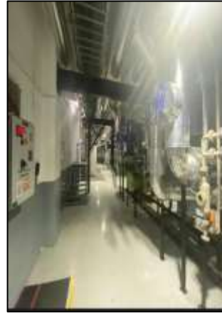
Internal View of Plant Room Tower 4, 5 & 6
