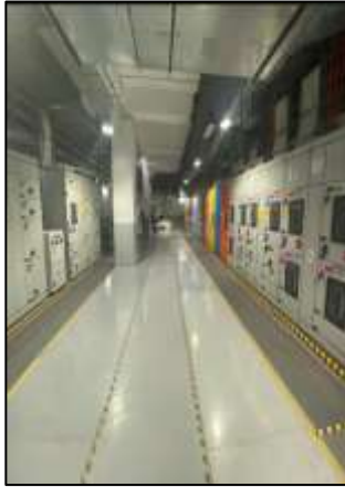
View of DG Room Tower 4 ,5 & 6
